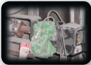
Fuel Air & Aux Air Drives
